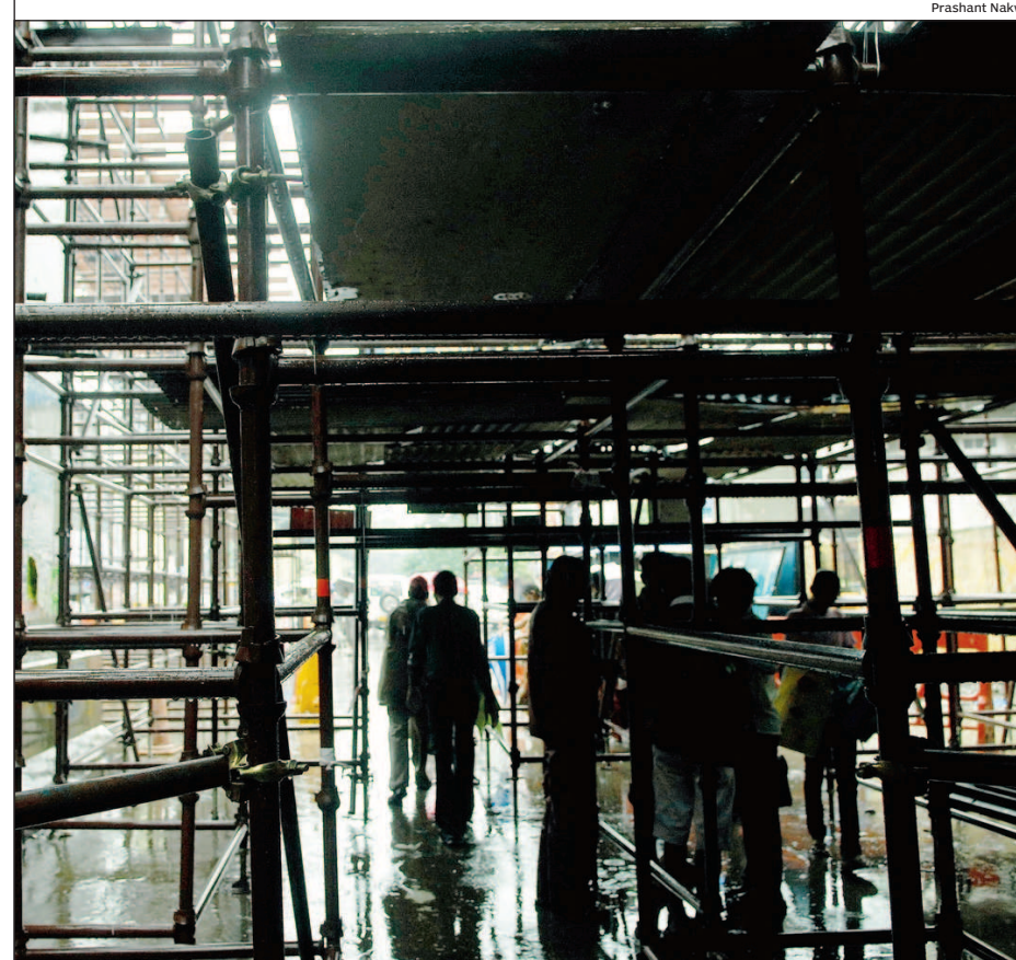
WORK IN PROGRESS: Work in full swing to connect the Metro corridor to the central railway and the skywalk near Ghatkopar station
